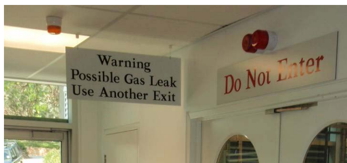
Warning signs and strobe lights
